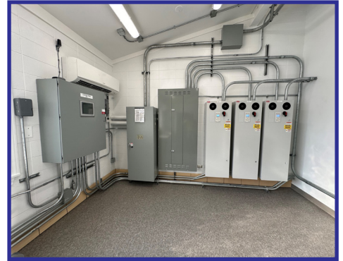
SCADA Control Panel & Pump VFD Controllers
